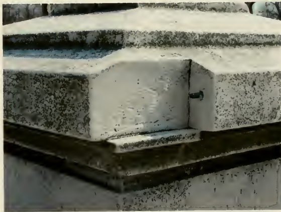
Figure 26: Missing dutchman repair and exposed metal pin
